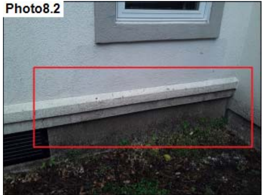
Impact damage thru-out
