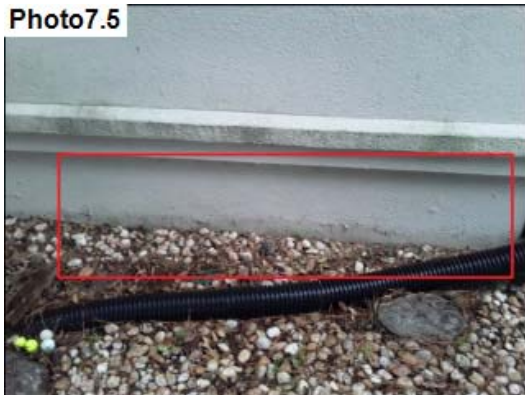
Foundation paint peeling off
