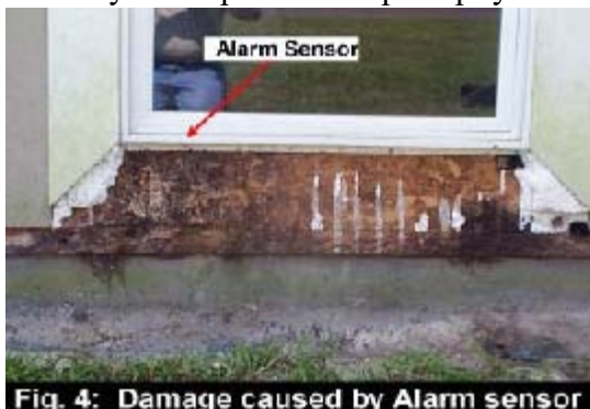
Fig. 4: Damage caused by Alarm sensor
