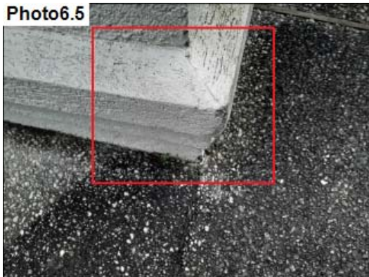
Impact damage at front corner of water table band
