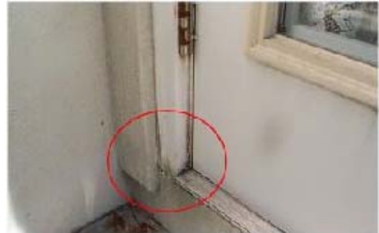
Fig. 1: Damage caused by No sealants
