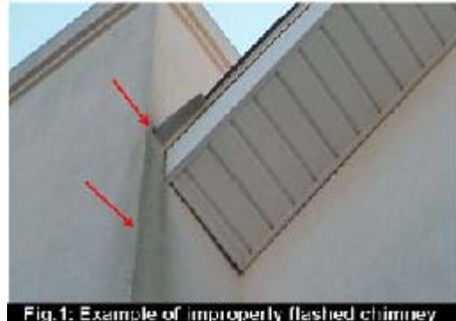
Fig.1: Example of improperly flashed chimney
