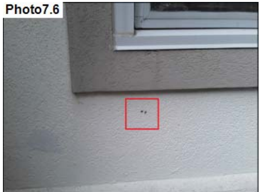
Previous inspection holes not sealed
