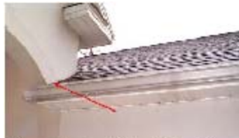
Figure 1: No kickout flashing
