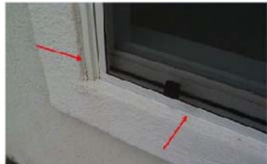
Fig. 2: Example of unsealed window perimeter
