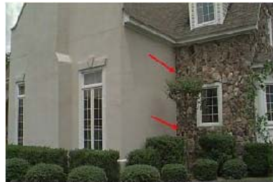
Fig.2: Stucco to stone needs to be sealed
