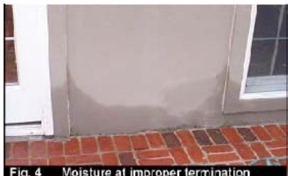
Fig. 4 Moisture at improper termination
