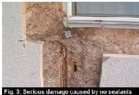
Fig. 3: Serious damage caused by no sealants
