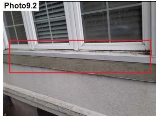
Some windows need resealing
