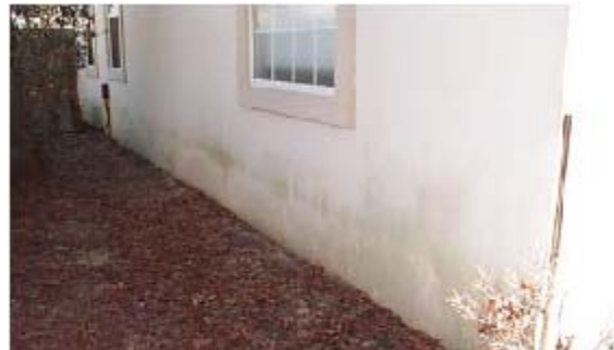
Fig. 1 Moisture caused by the wicking process
