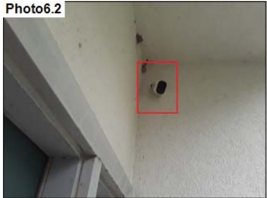
Hole behind the camera needs to be repaired.
