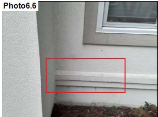
Impact damage at water-table band
