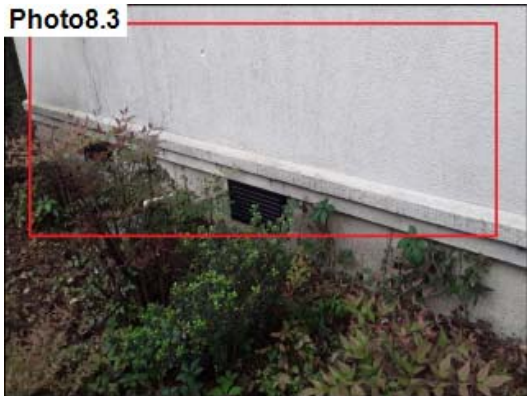
Impact damage and vegetation on lamina
