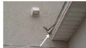
Fig 2: Improper installation (unsealed)
