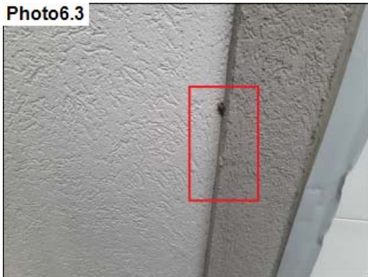
Impact damage and exposed mesh
