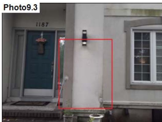
Repair needed where railings were removed
