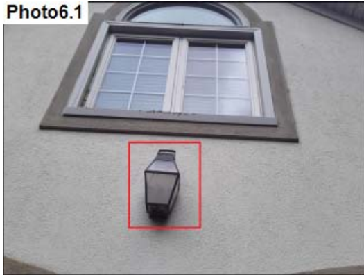
Compression Crack Light Fixture needs to be sealed
