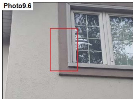
Impact damage and compression crack
