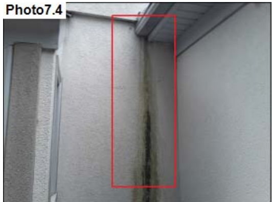
Mildew & stains from roof
