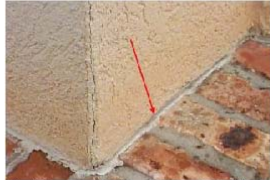
Fig.1: Stucco to brick transition needs sealing
