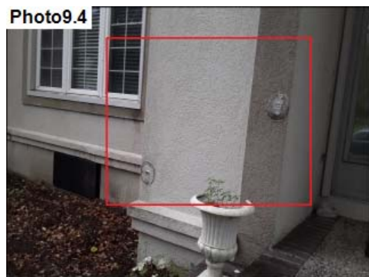
Repair needed where railings were removed
