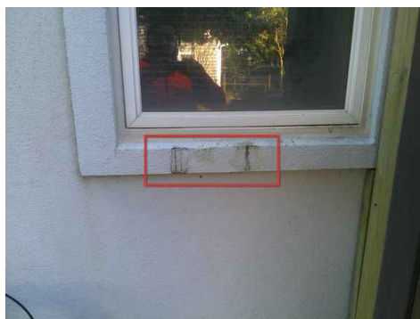
Cracks / Impact Damage
