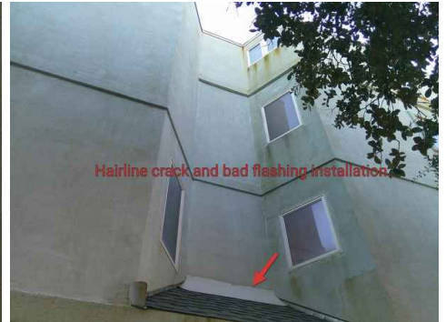
Hairline crack and bad flashing installation.
