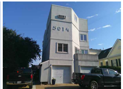
Lamina needs resurfacing.
