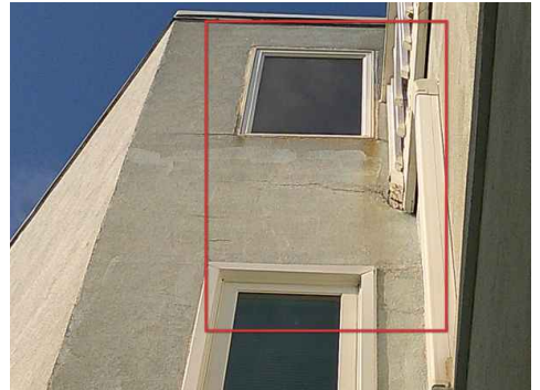
Moisture intrusion from cracks and terminations.
