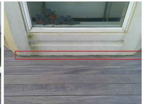
Improper Deck Flashing and Impact Damage
